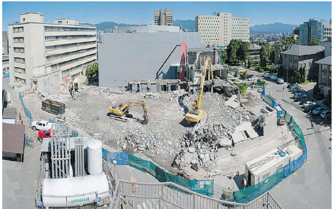
Construction of VGH's Joseph &amp; Rosalie Segal Family Health Centre is one project designed to build a healthy and sustainable future in B.C.
